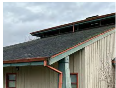
Roof appears to be end of life
